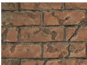
Fire Cracked Brick
